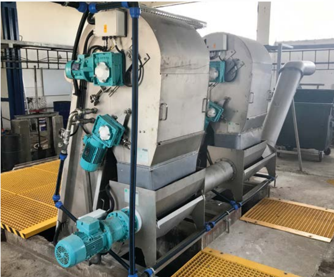
WWTP, Stupava, Czech Republic, 800_CP_1050 + LS_2400
