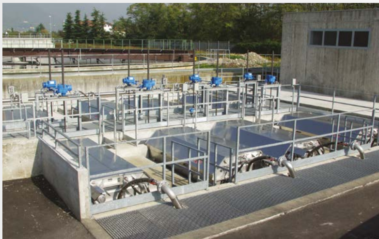
WWTP, Italy, 6FBB
