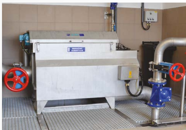
WWTP, Czech Republic, 2FBO
